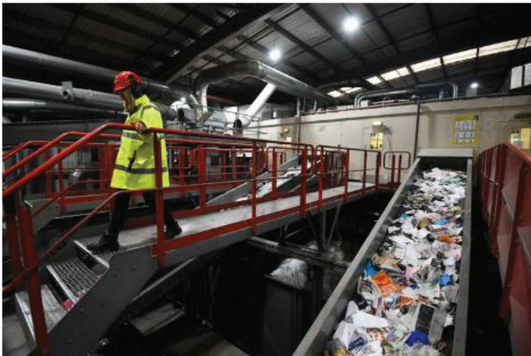
The proposed new alternative energy facility could take in black bin waste from all over the UK, including South Holland. Stock image.
